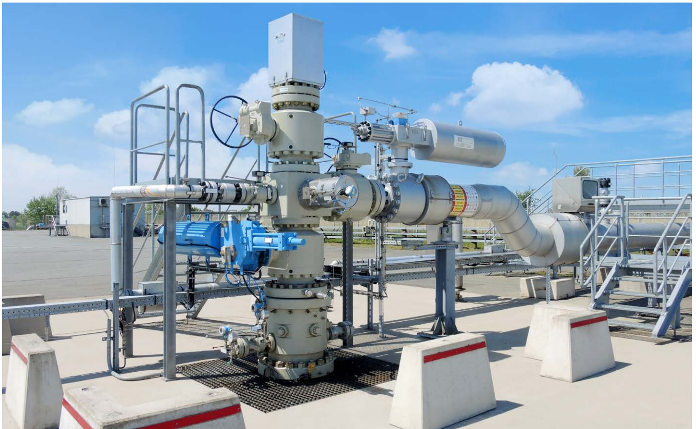
State of the art: gas cavern well heads in Etzel
